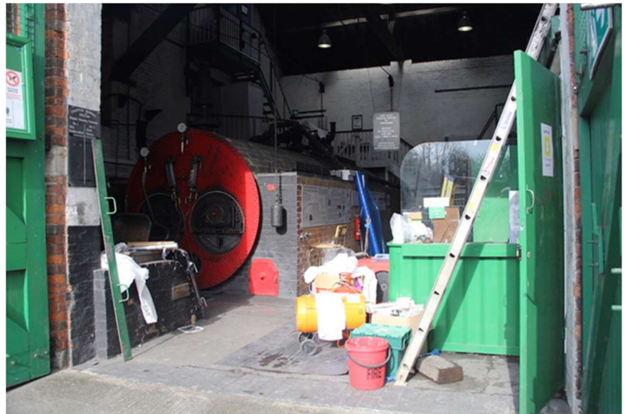
The Steam Boiler
