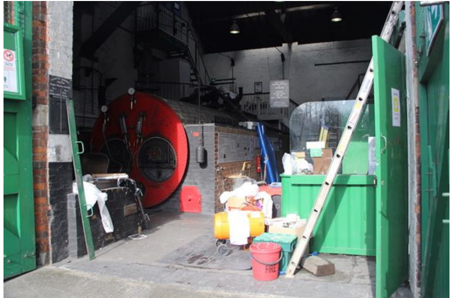
The Steam Boiler
